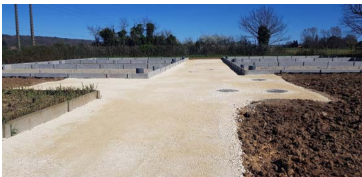
Station Epuration St Germain et Mons
